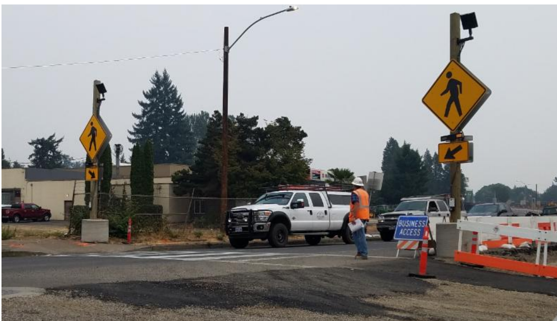
Temporary Rapid Flash Beacon helps pedestrians cross the road
